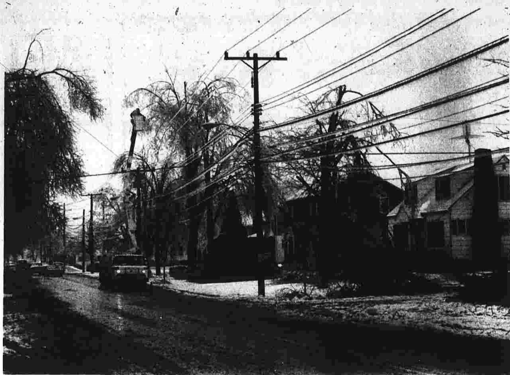
Power company repair crews work on W. Middle Tpke. near Alton St.
